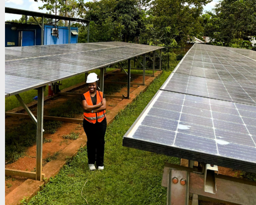
Eliane Nirere at a KUDURA Power solar mini-grid system in Kenya. Photo courtesy of Nirere
